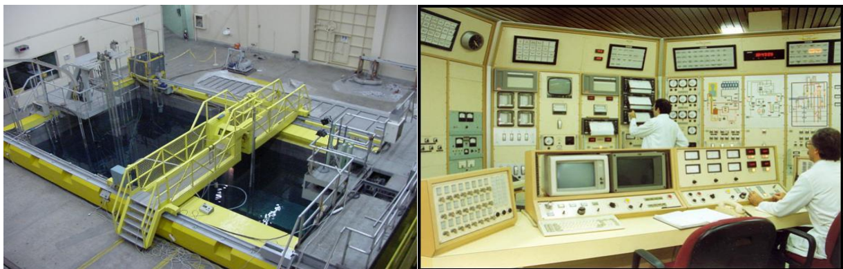
Figure 2. TR-2 Research Reactor
